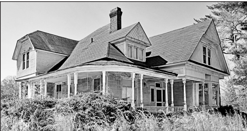
August 2023, The state of the historic house after being purchased from the Nelson family, descendants of J. Miles & Maggie Berrong. Photo Credit: Bruce Roberts
